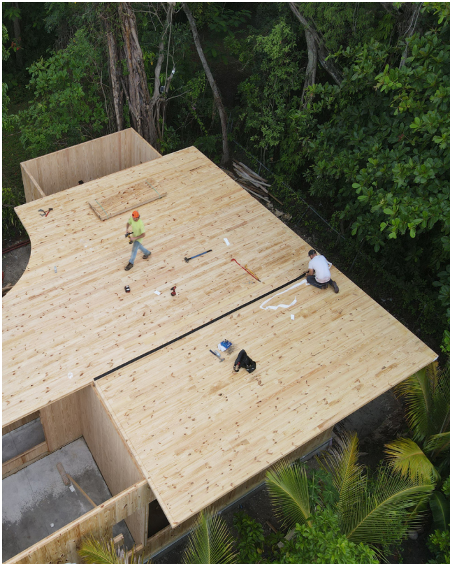
Figure 5. In process construction photo of the first CLT structure to be permitted and erected in Miami-Dade County. Image by Atelier Mey.
